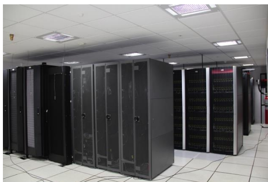
Figure 3.3 CSIR centralized 489 TF High Performance Computing Facility
