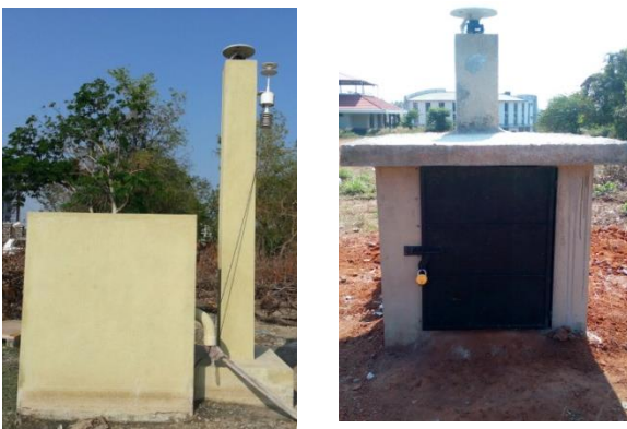
Figure 5.3 CGNSS stations established in Chennai and Udupi respectively
