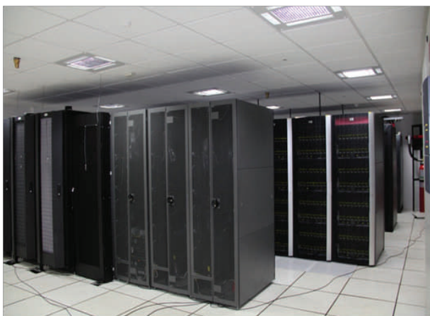
Figure 4.6 CSIR centralized 360TF High Performance Computing Facility.
