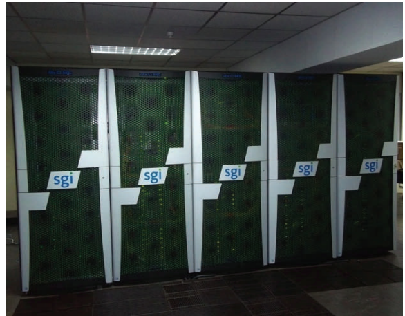
Figure 4.8 Altix ICE system with 2304 processing cores distributed over 192 nodes and 30 TB of parallel file system along with all associated hardware and software.
