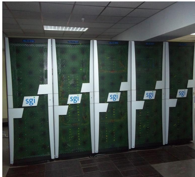
Figure 4.7 Altix ICE system with 2304 processing cores distributed over 192 nodes and 30 TB of parallel file system along with all associated hardware and software.
