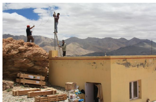
Figure 1.1 Installation of the instruments with the weather sensors at IAO, Hanle in Ladakh. Inlet fixed on the top on the building
