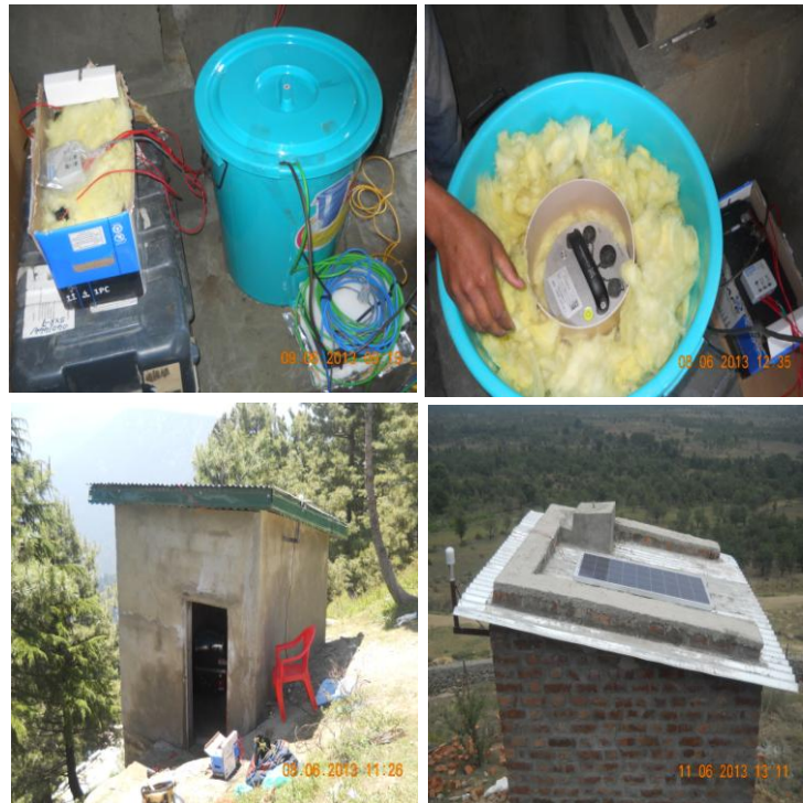
Figure 6.21 The housing of broadband instruments and installation of equipments
