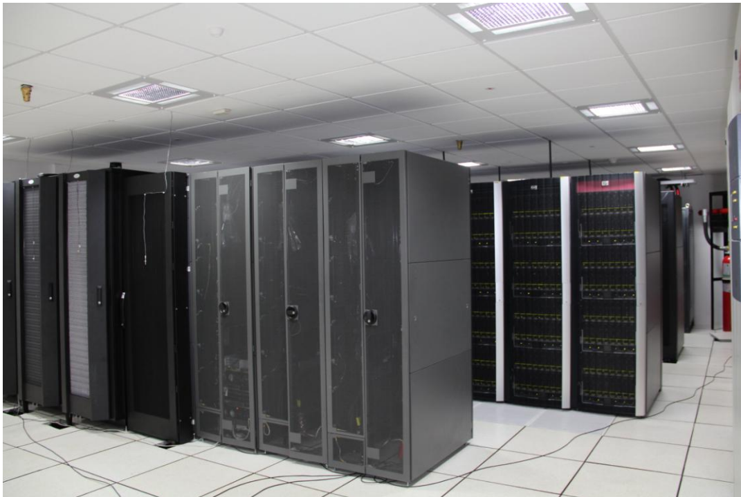
Figure 4.6 CSIR centralized 300TF High Performance Computing Facility. The system consists of 22 numbers of 42U racks with 1088 nodes with more than 2 Peta Byte of usable parallel file system.
